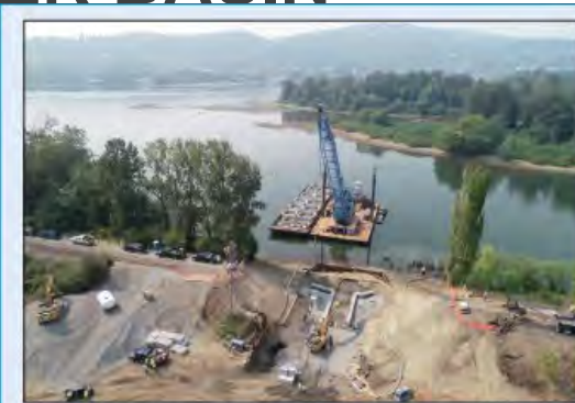
Photo courtesy of U.S. Army Corps of Engineers, Portland District Aerial view of construction at Oaks Bottom Wildlife Refuge – the largest remaining natural area in the lower Willamette River floodplain.
