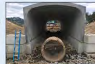
The project replaced an old pipe culvert, pictured here in the front of the new salmon-friendly box culvert.
