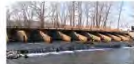
Fig. 2. Bannister Ford over Little Niangua River is a significant barrier to fish passage and a priority for replacement.
